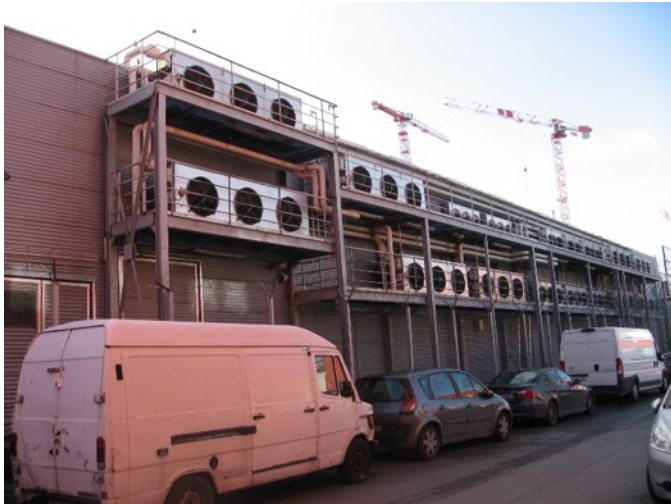
Interroute/Interxion St Denis
